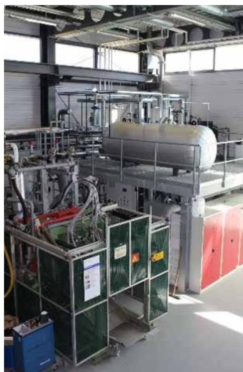
High-pressure steam supply (manufactured by BBS) at Fraunhofer ICT.
